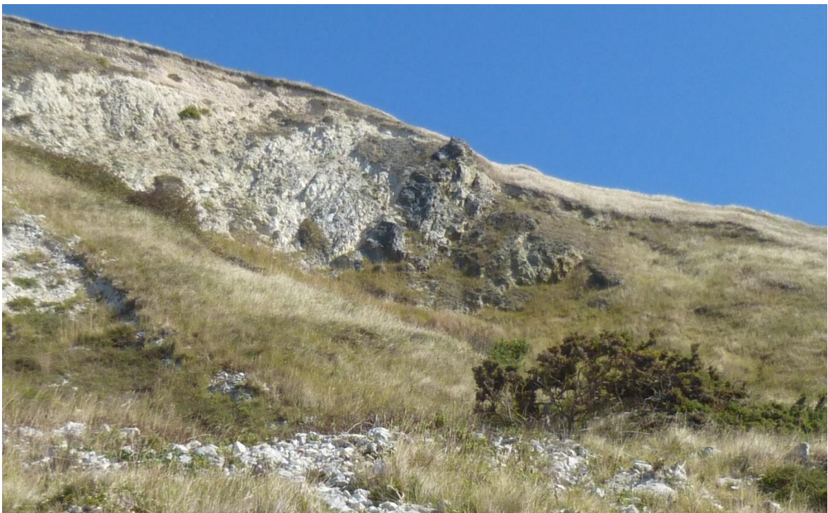
Junction between the Greensand and the Chalk with a large landslide sliding on the Gault clay and covers the lower greensand
