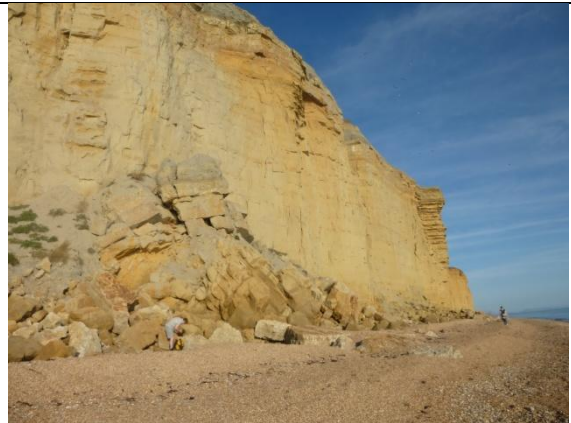
Landslip of fullers earth and underlying inferior oolite
